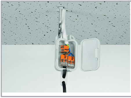
Pendant light connection in a suspended ceiling
